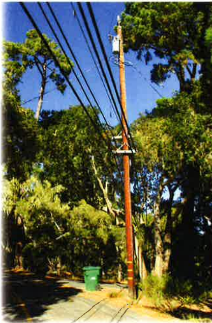
These high voltage electrical and communication lines no longer snake through the trees in our Phase One project area. Undergrounding will increase service reliability and reduce Forest-wide outages caused by storms and falling branches.
