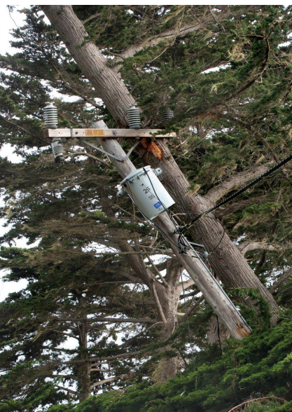
A toppling tree leans against an electrical transformer in the forest after a February 2019 storm.
