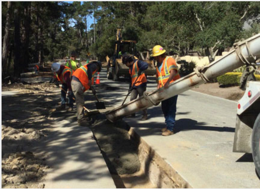
Left: Underground utility crew from contractor Leo Tidwell Excavating Corp placing concrete slurry cap over newly installed conduits along Forest Lake Rd. as part of the Phase 3 Undergrounding Overhead Utilities Project.
