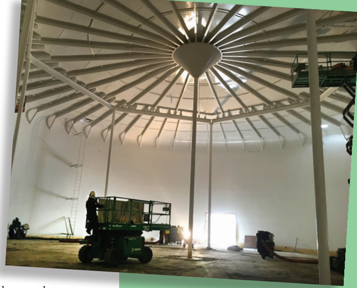
The newly renovated Poppy Hills storage tank (shown above) is part of the District's recycled water distribution system, which also includes Forest Lake Reservoir and seven miles of pipeline.
